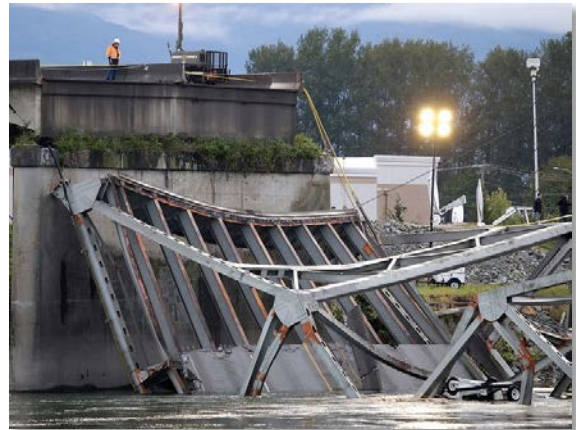
When the bridge goes, so does the water main and communication lines attached to it.
